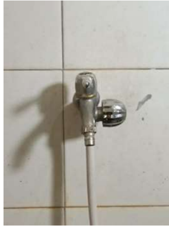
Figure 7. Water Faucet in the Bathroom
