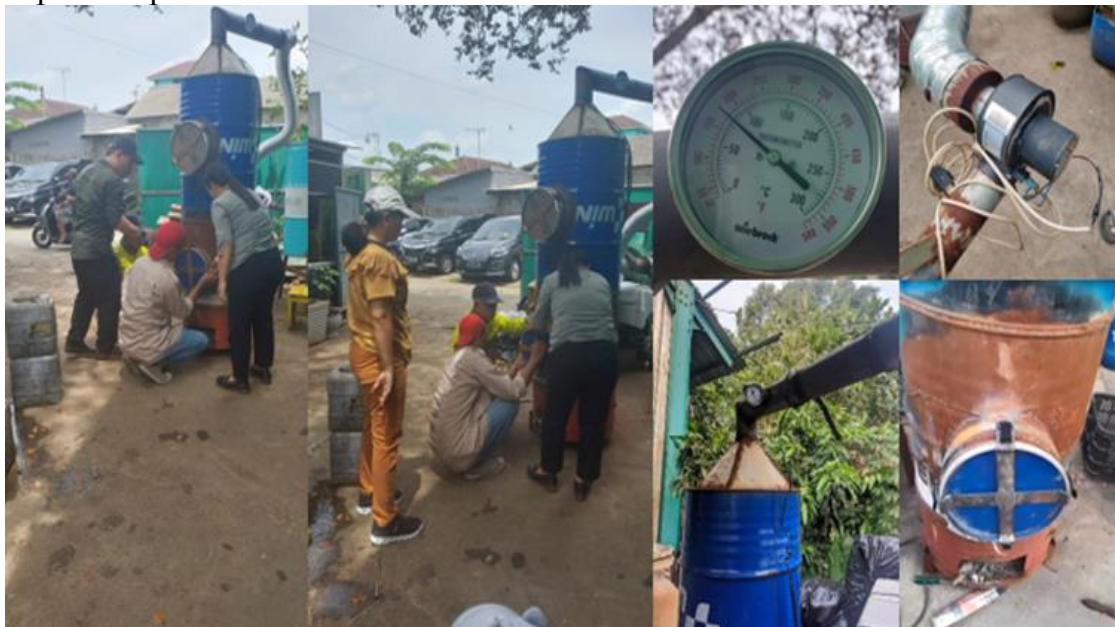
Figure 4. The PkM Team Conducted a Re-Inspection of the Repaired Organic Waste Incinerator
