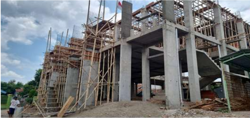
Figure 6. Condition of the Mosque
